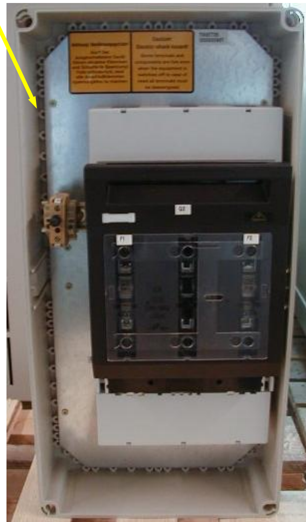
Battery fuse box
